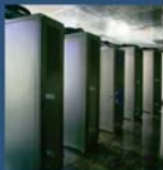
Texas server room
